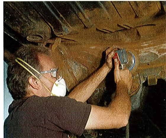
While the suspension and gas tank were out, it was a perfect time to clean up the bottom of the car and get it ready for a coat of paint since the front half has already been tended to.
